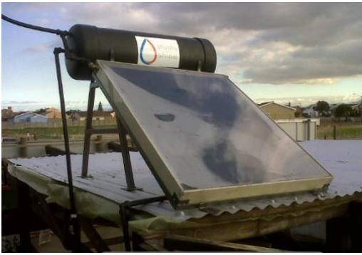
Fig. 3: The Solar water heater installed at a community centre (courtesy of CPUT: Mech. Eng. Dept.)
